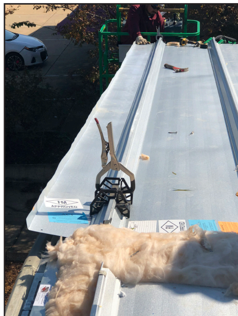
Installed Termination Panel
