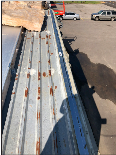
Termination with High Capacity Rake Plate Upslope View
