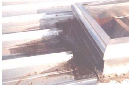
This curb has no clearance on the upslope end, which allows a water head to build up.
